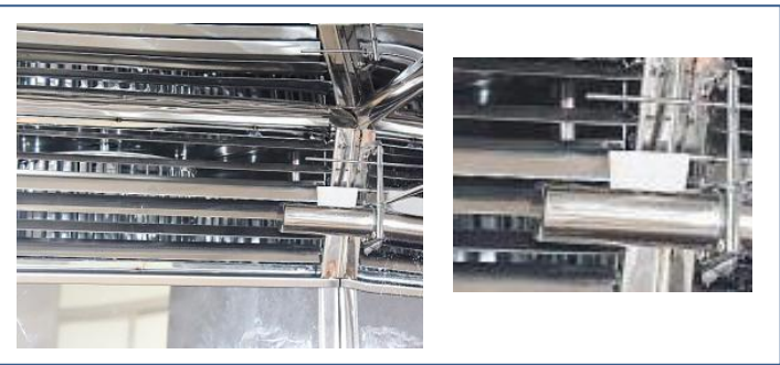
Temperature and Humidity Sensor
